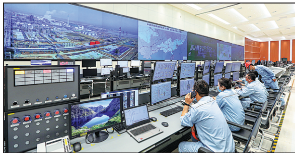
Engineers use digital technologies to monitor operations at Zhongke (Guangdong) Refinery and Petrochemical project in Zhanjiang. ZHANG FENGFENG / FOR CHINA DAILY
