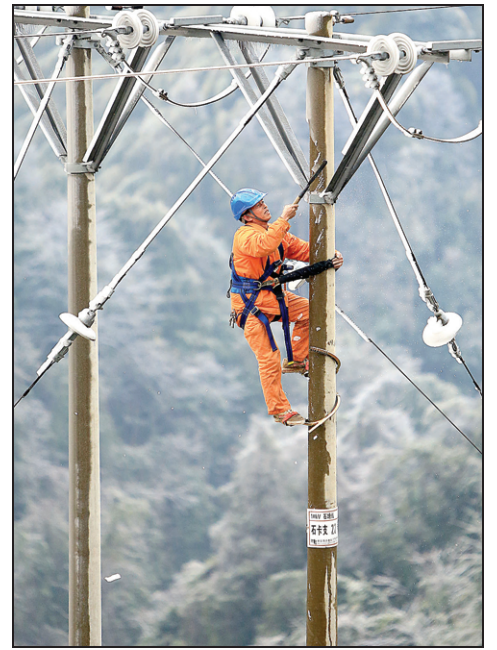
A worker maintains electricity transmission lines in Liuzhou, the Guangxi Zhuang autonomous region.
